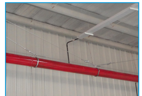
Bracing for steel pipes
