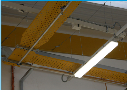
Busbar and Lighting
