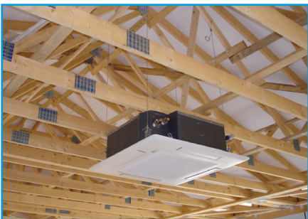
Air conditioning units
